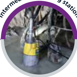
Water Recovery / Intake
